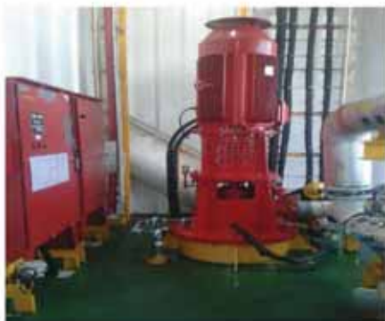
海洋平台(锦州9-3)电动消防泵 Offshore platform(Jinzhou 9-3) electric-drive fire pump
