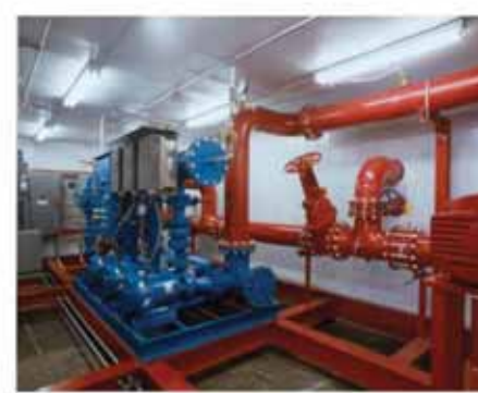
孟加拉AKG水处理站工程 Bangladesh AKG Water treatment station project
