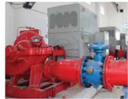
扬子石化电动消防泵 Yangzi Petrochemical electric-drive fire pump
