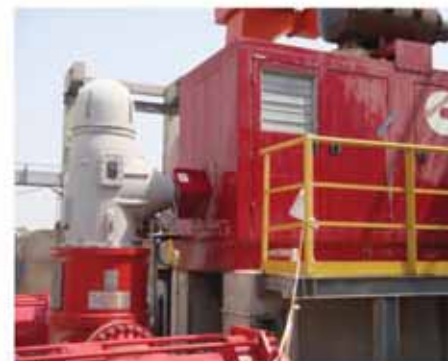
柴油机海水消防泵 Diesel engine seawater fire pump
